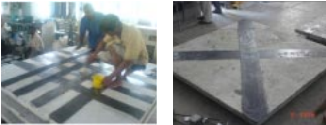
Different Patterns of Using Carbon Fibre Wraps in Corrosion Damaged RC Slabs for strength Restoration
